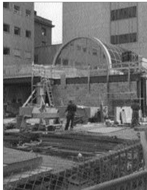
The plaza construction progressed over the summer, with a fountain area and an accompanying grass grove. Photo by Pavani Thagirisai.
