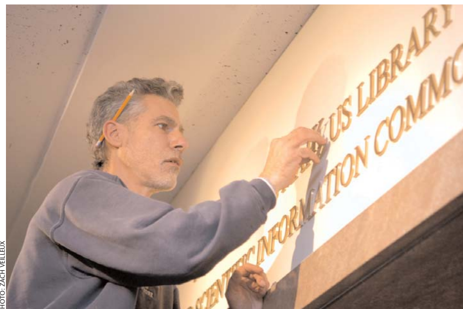
Hallowed halls. A workman installs new lettering above the entrance to Welch Hall, acknowledging Rita Markus's contribution to the university's library.
